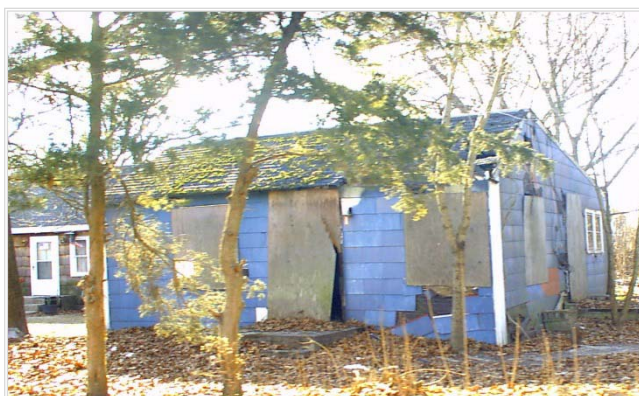
Severe housing blight on Old Quogue Road in Riverside
